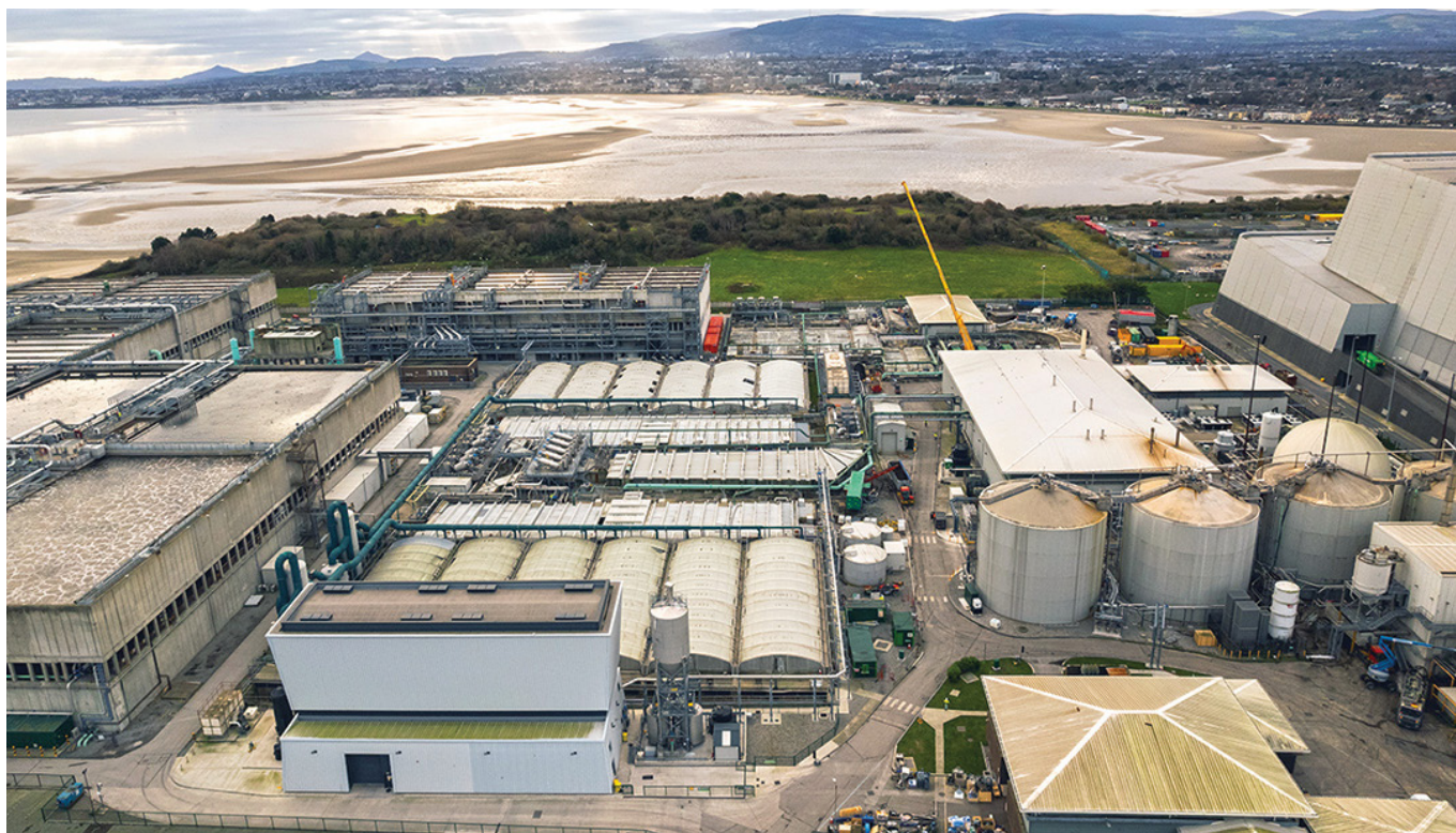
Sludge processing facilities at Ringsend Wastewater Treatment Plant, Dublin, Ireland's largest sludge processing facility. Image courtesy of Murphy.
